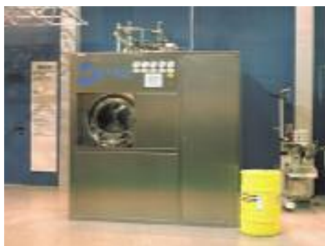
Figure 5: Facility for laundering work clothes (LANL, USA)
